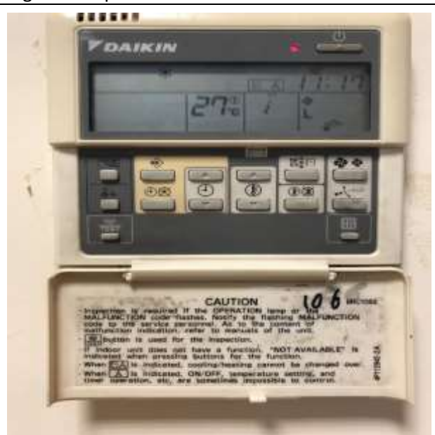
Climate control panel
