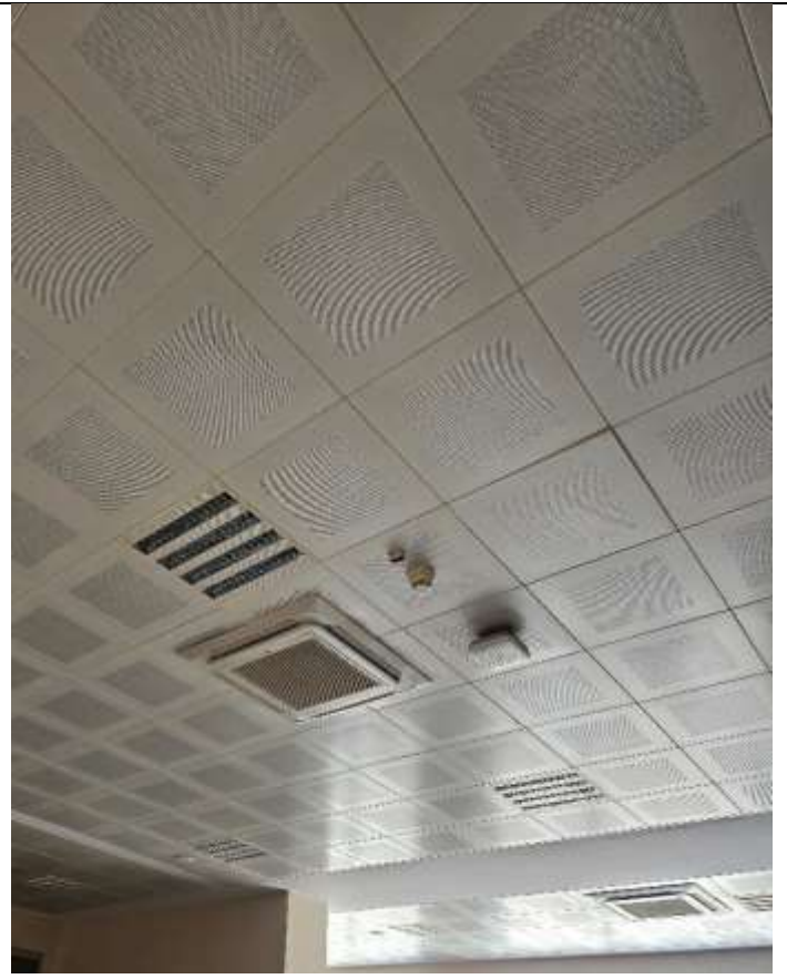
Thermal comfort, Air quality monitoring systems with fire detectors
