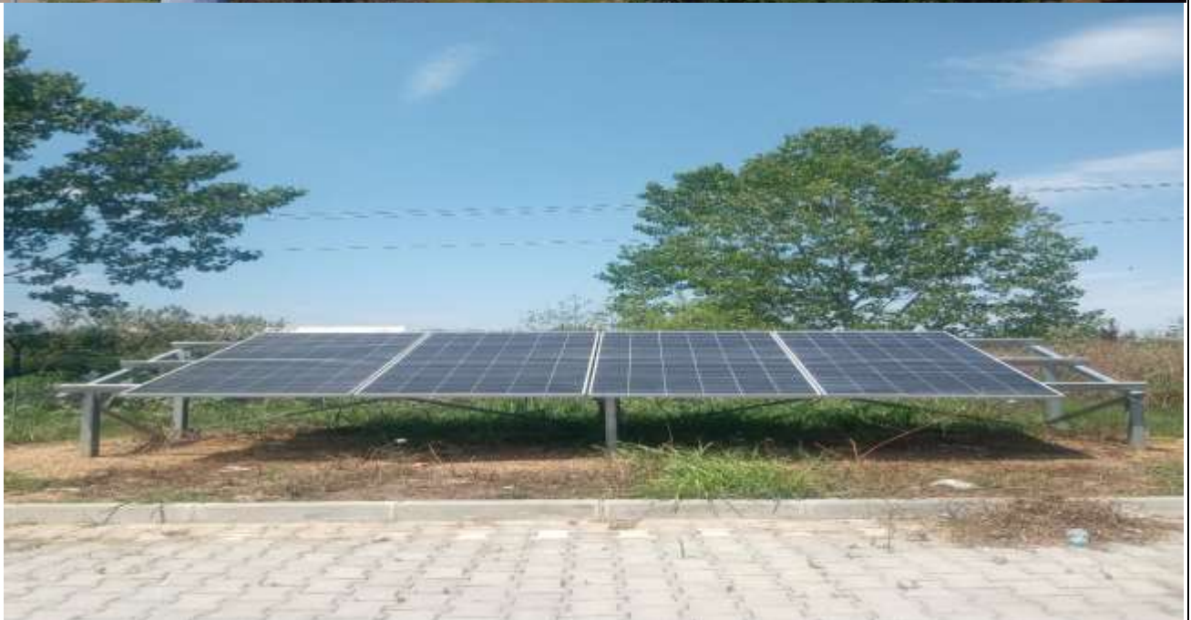
Solar Panels (Gebze Technical University, Türkiye)
